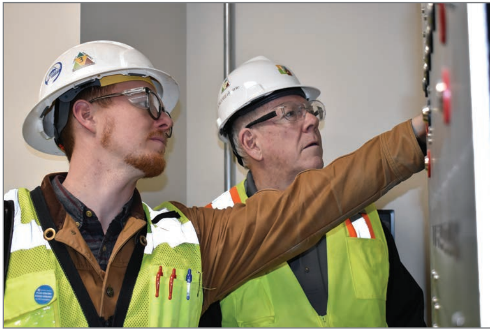
Engelstad and McGovern examine a fire alarm station to ensure proper installation.
